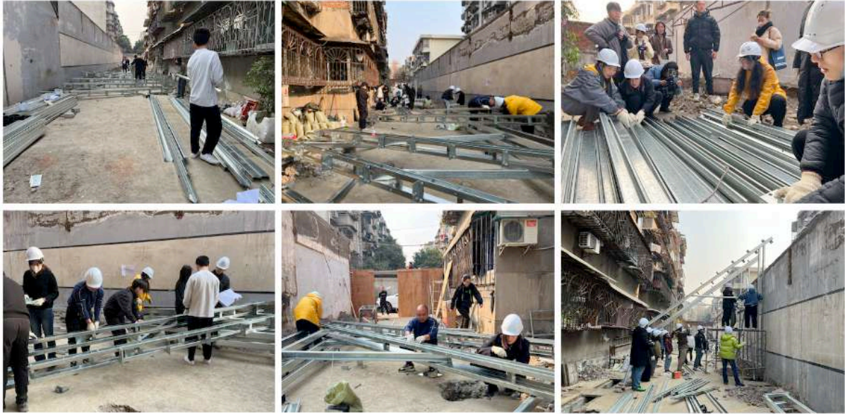
Fig. 6-7 Process of construction with participation of all project members, the party secretary of local community and several residents, under supervision of two structural engineers
