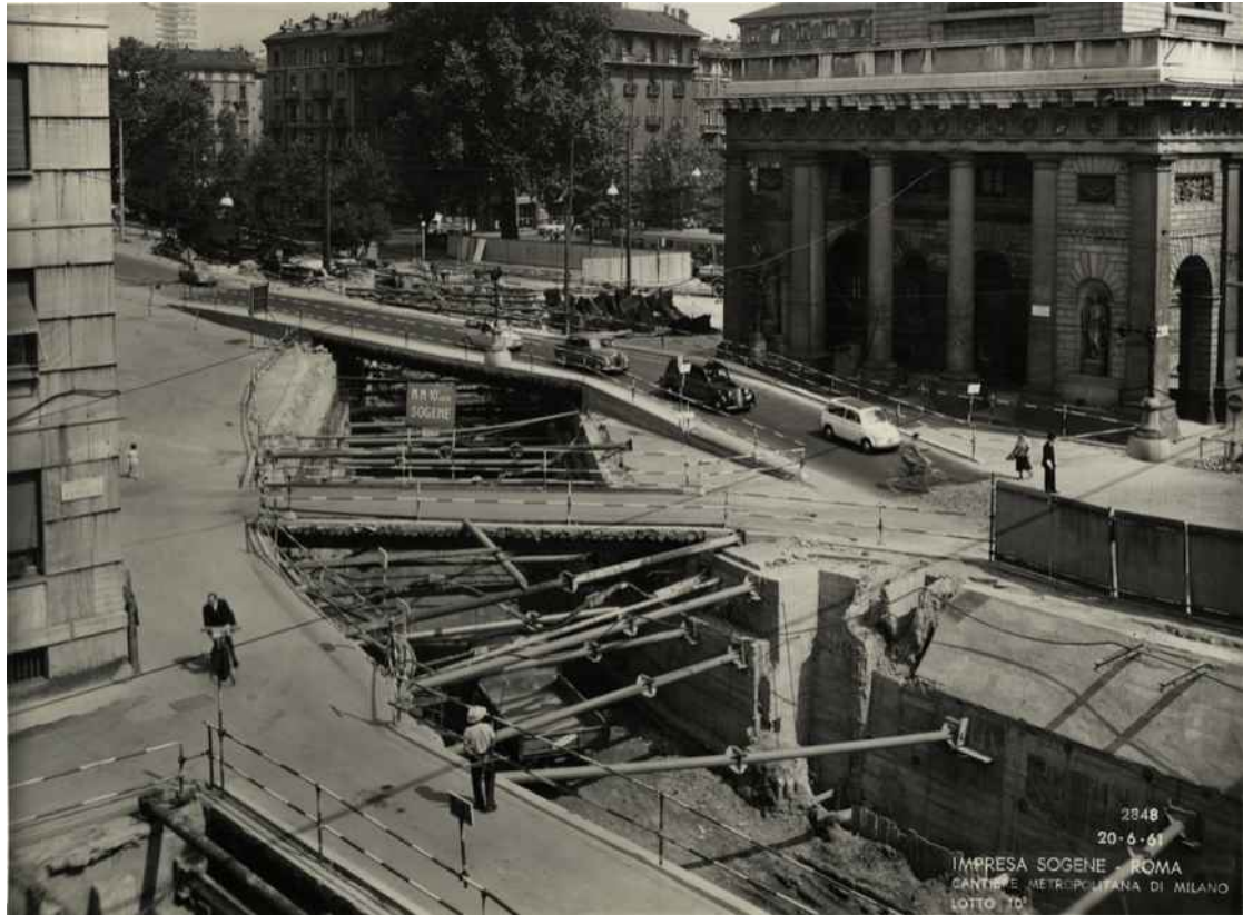
Fig. 6.7 – Construction work to build the metro in Porta Venezia covering the Cavo Redefossi; source: Urban File.org, online
