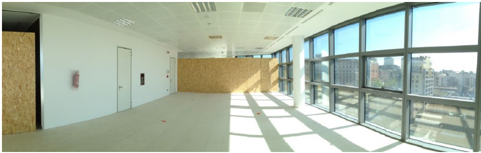
Figure 2. View showing the partial height OSB sheets (center and left) which partition off volume V_2 from the main volume V_1 and from the rest of the volume.
