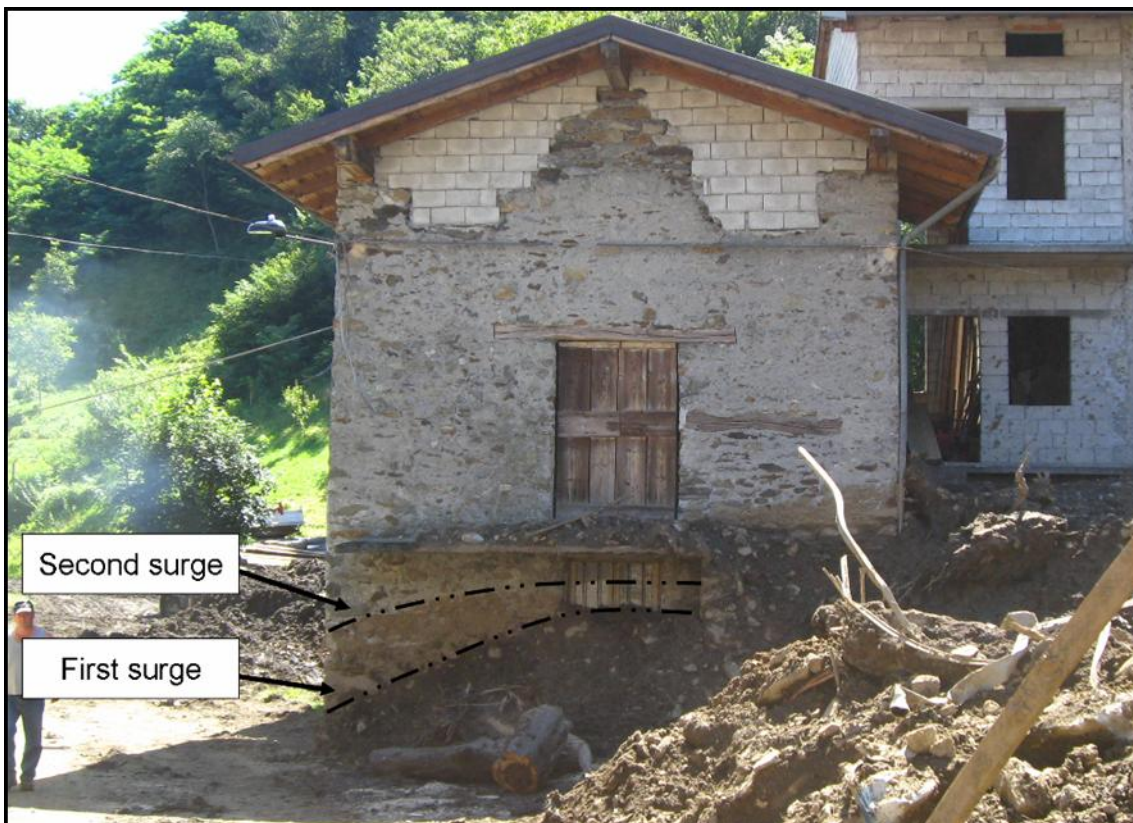
Fig. 10.5 – Deposit traces left by the flow on one of the houses situated in the alluvial fan of Selvetta. The two surges of the flow can be distinguished. Photo J. Blahut.
