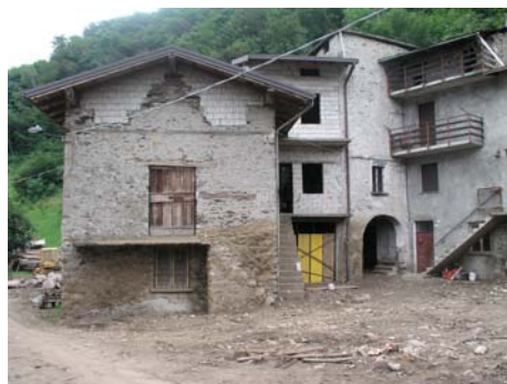
Fig.5. Buildings damaged by the landslide of July 2008 in Colorina, Sondrio
