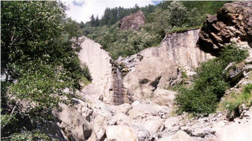
Fig.5. Example of non efficient dike (broken in the central part), Lanzada (Sondrio).
