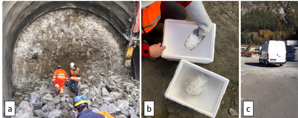
Figure 4.4: Frozen blocks recovering: a) directly from excavation face during excavation with a hydraulic hammer; b) dry ice added to avoid melting of pore-ice; c) isothermal van used to bring blocks to San Gerardo Hospital.
