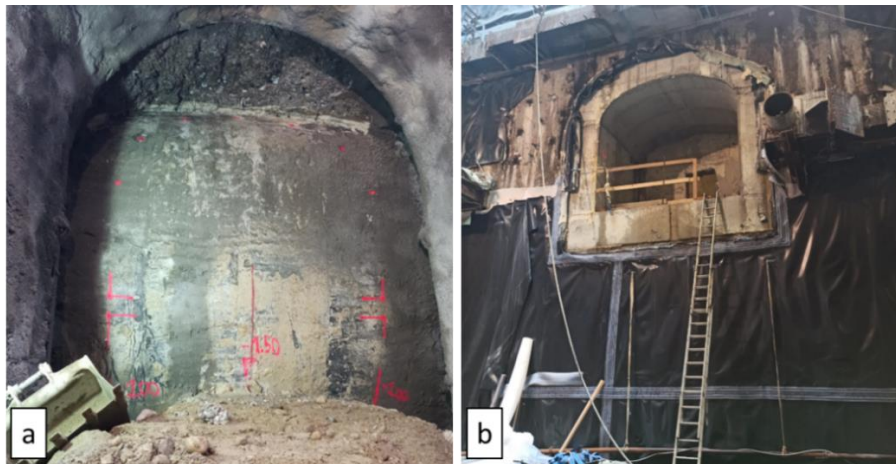
Figure 1.18: Lining of cross-passage: a) temporary lining of shotcrete merged to the external surface of tunnel concrete lining bored by TBM; b) definitive concrete lining of cross-passage, view from shaft.
