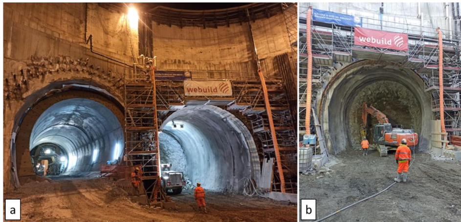
Figure 1.15: Excavation activities: tunnel excavation also continues at night from the north shaft P4 and b) is also carried out simultaneously from the opposite direction (south shaft P2).
