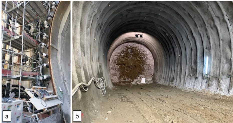
Figure 1.16: a) External portion of freezing pipe working during maintenance phase; b) temporary lining made by iron ribs covered by shotcrete on sides and crown, at the end frozen soil shell is notable.
