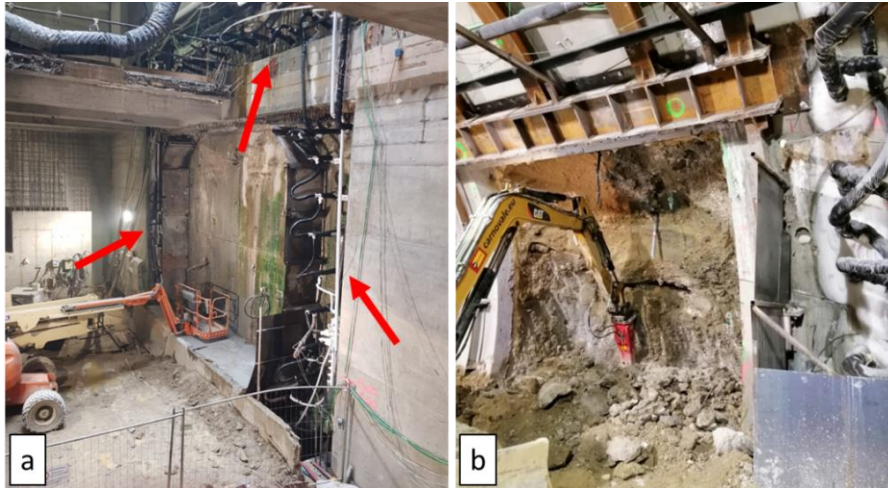
Figure 1.17: a) Installed freezing pipe from DW; b) demolition of diaphragm and excavation of frozen soil by hydraulic hammer.
