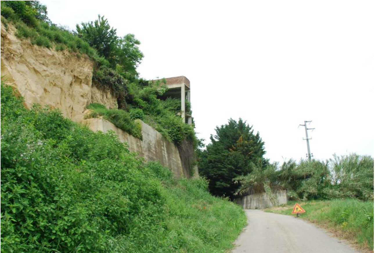
Fig. 27 First SH landscape. Unfulfilled promises of building expansion. The skeleton of a new building in a state of disrepair. The road, with direct access to the centre of the village, is damaged by hydrogeological instability of the hill above. Nature has taken over the no longer cultivated fields.
