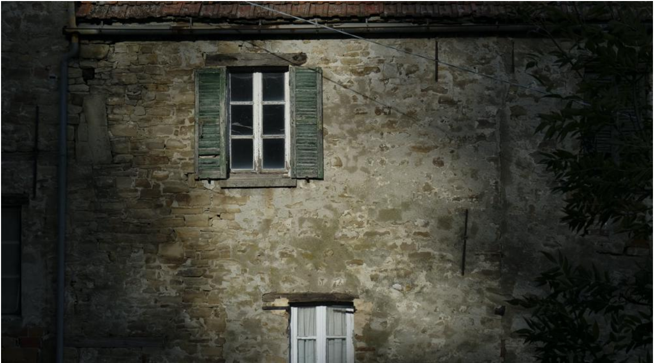
Fig. 42 Fourth SH Landscape. Stone façade in a building in the historic centre. The house is in a state of neglect, like many others in the historic centre. Despite its central location, it does not have access to basic services, which are not present in the village.
