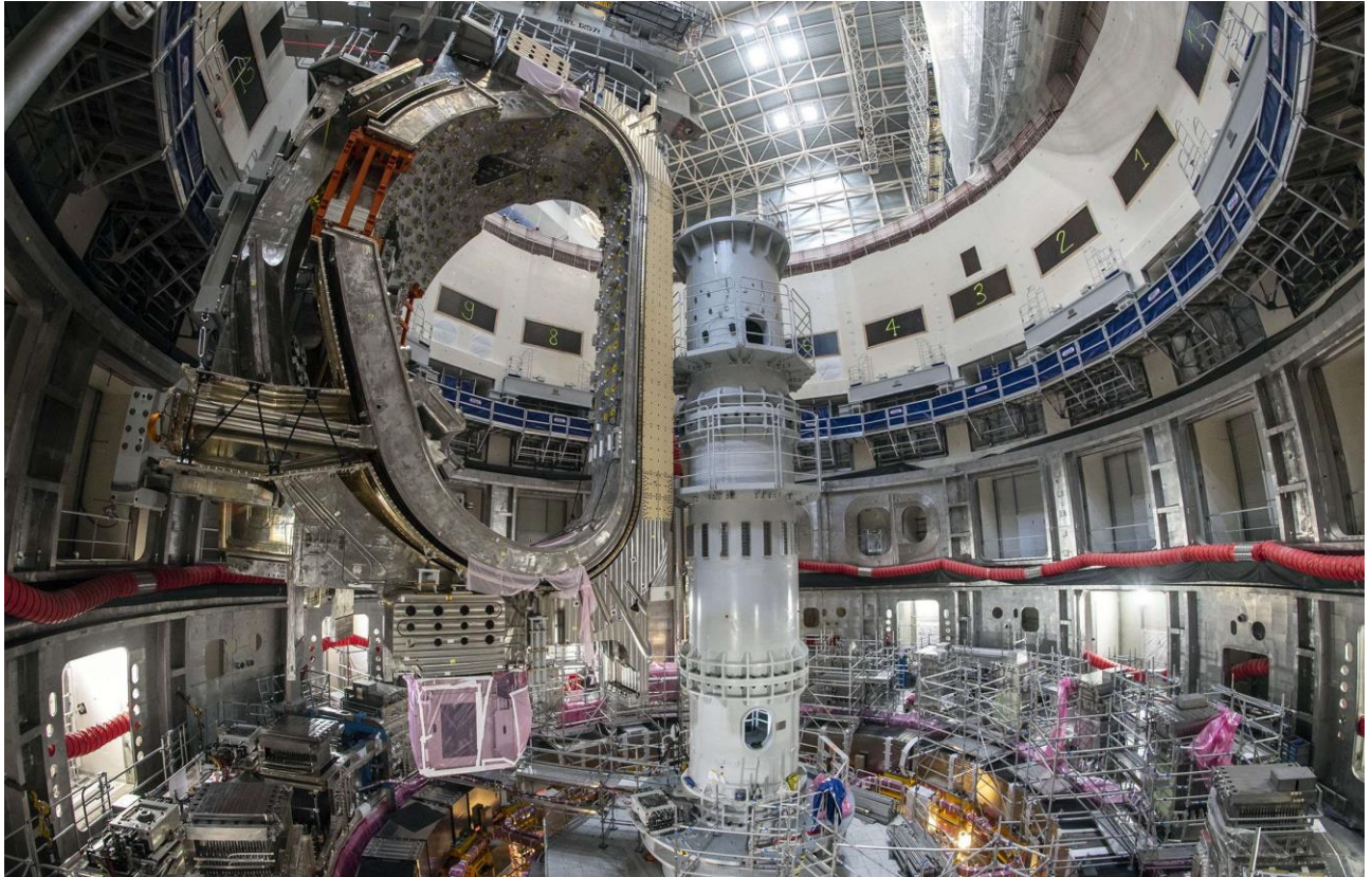
Figure 1.11: Picture of the chamber in which ITER is installed, taken in 2022. On the left one section of the torus is being put in place.
