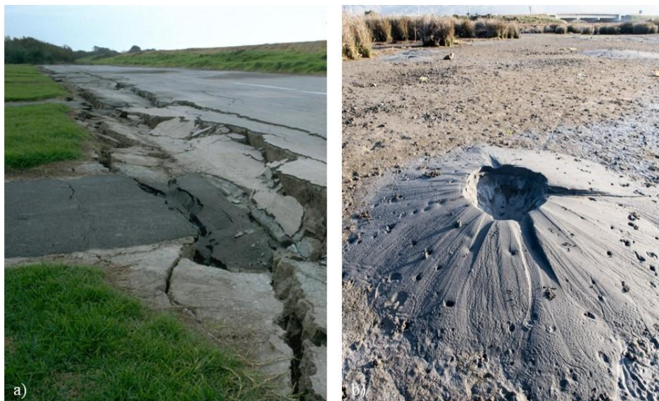
Fig 1.3 Effects of liquefaction: a) Lateral spread; b) Sand boils
