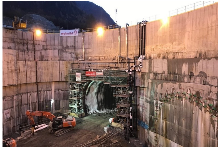
Fig. 7-7, Artificial ground freezing with closed system technique (AGF-BR): maintenance stage with brine during the excavation of a railway tunnel for the underpassing of the Isarco River (Brenner Basis Tunnel site – 2021)
