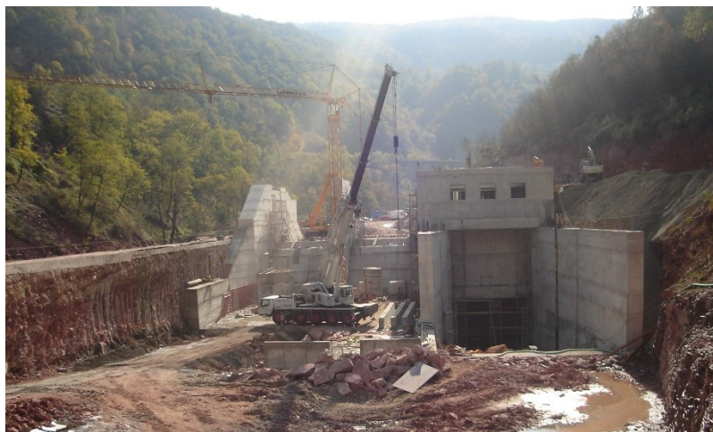
Fig. 7-5, A vertical jet grouted wall (on the right) made with the double fluid system, performed from the crown of a river diversion embankment to protect a hydro power plant construction
