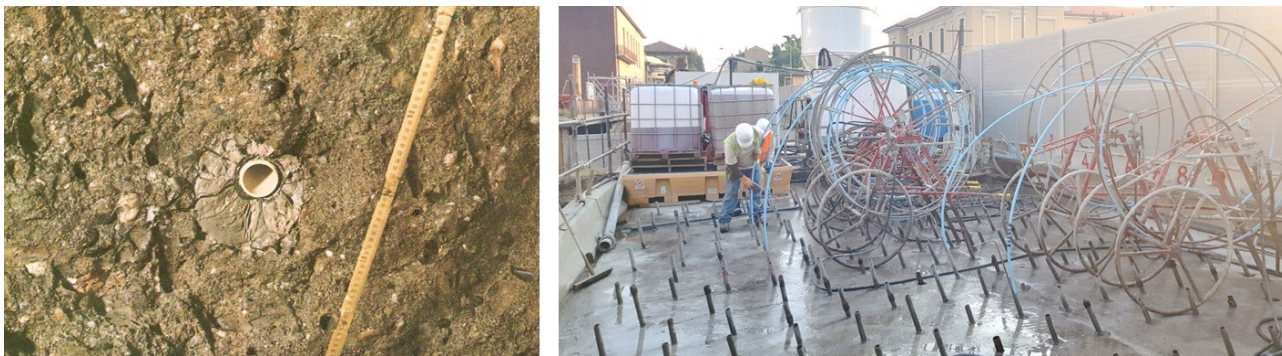
Fig. 7-3, Permeation grouting practice - Left: TAM in correspondence of a manchette, surrounded by the cement-based sheath, into the treated soil (Rodio) – Right: TAM grouting phase on site (Milan Metro Line 4 site – 2019).
